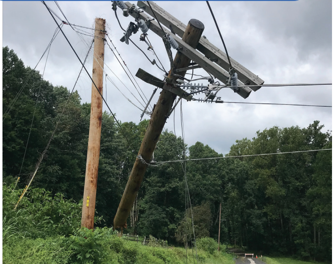
Damage across Southern York County affected the co-op’s electrical system, taking down poles and wires as the storm passed through.
