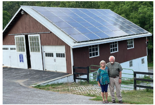
SUNNYSIDE UP: Members Mary and Ed Franco show off their rooftop solar array, located in our Shippensburg District.
