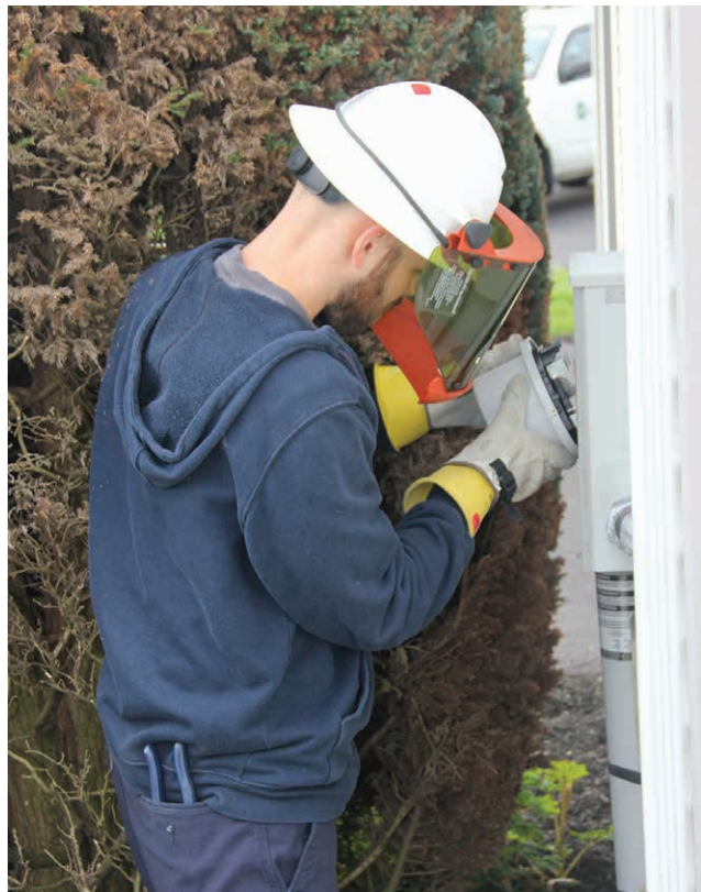
UPGRADING: Adam Willman, field services person B for Adams Electric Cooperative, exchanges a meter at a residence in Gettysburg as part of a system improvement project. All meters will be replaced over a five-year period.
