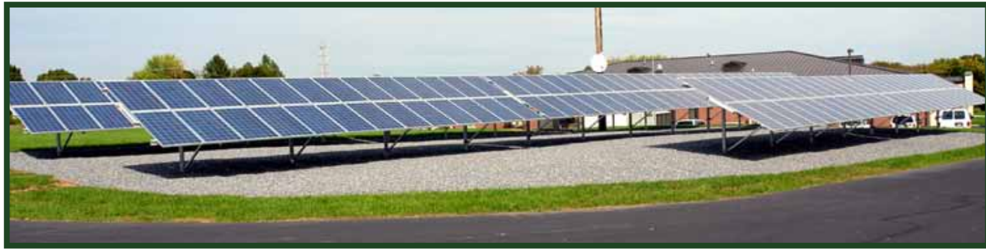
Adams Electric's Solar Generation: A 45.76 kilowatt photovoltaic system is located at the co-op's Gettysburg headquarters office. The 200-panel solar array system has exceeded expectations since it began operations in October 2010. To view the live generation reports, visit adamsec.coop and click on the Solar Dashboard button.
